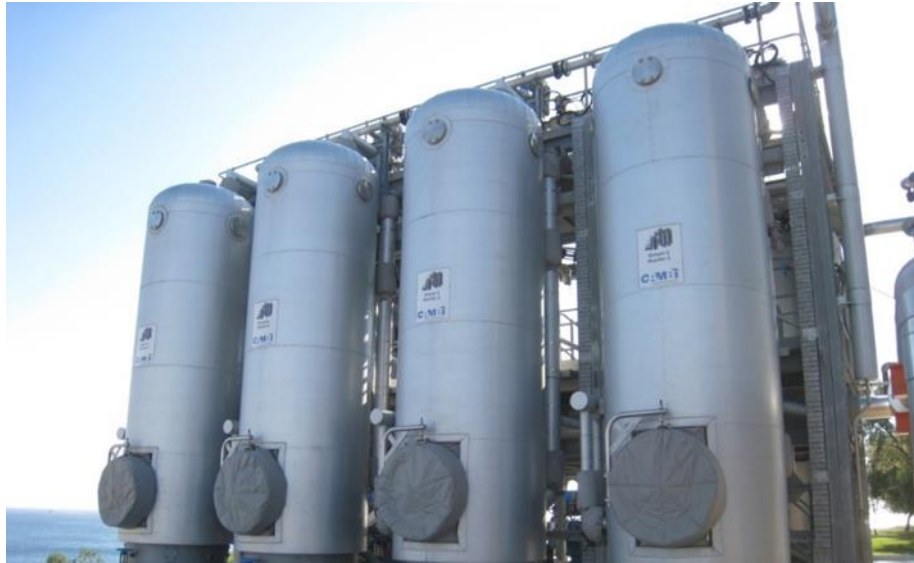
Figure 3: B6-4 thermal hydrolysis plant with 4 reactors at Psyttalia WWTP
