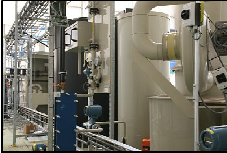
Figure 8: Full scale NutriTec ® concept for recovery of ammonia and phosphate from human urine
