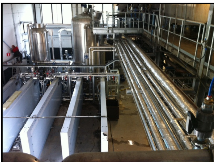
Figure 7: Full scale the TurboTec® thermal hydrolysis plant at WWTP Venlo
