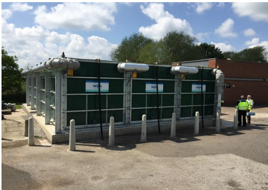
Figure 4: A 5,000 PE WPL Hybrid-SAF™ modular wastewater treatment plant installed at Site 1 in 2017.
