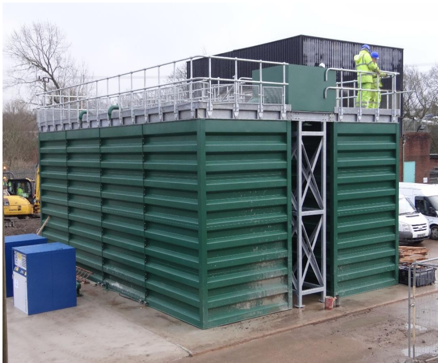
Figure 2: A 10,000 PE steel WPL SAF modular tertiary wastewater treatment plant.
