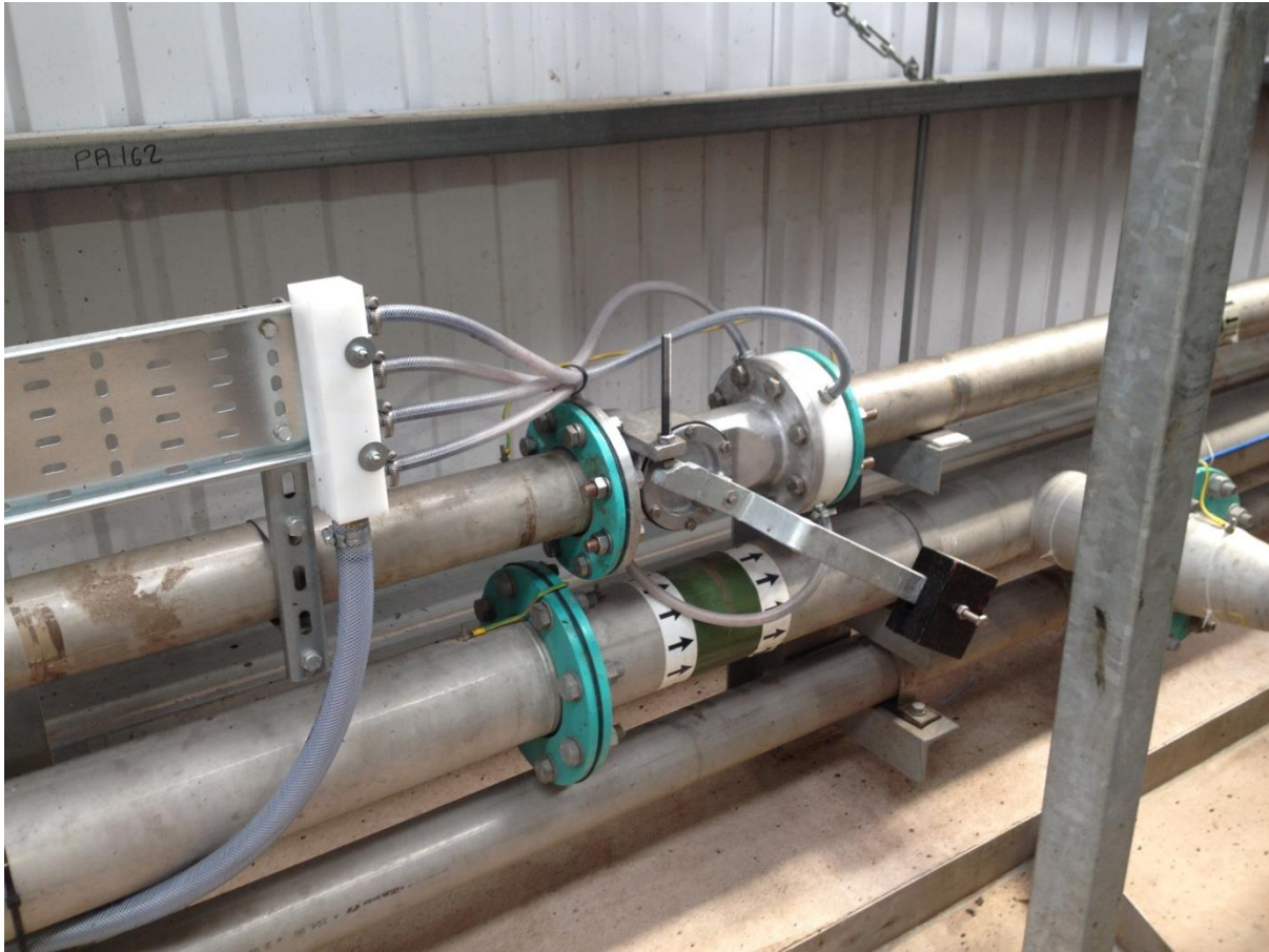
Figure 4: Polymer multipoint injection ring and mixing/shear valve on sludge feed pipe work
