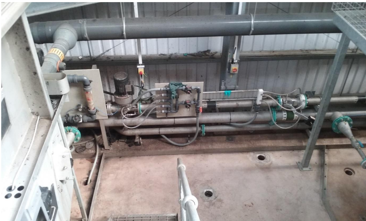
Figure 5: FloMix unit installed on plant between the mixing/shear valve and the flocculation tank
